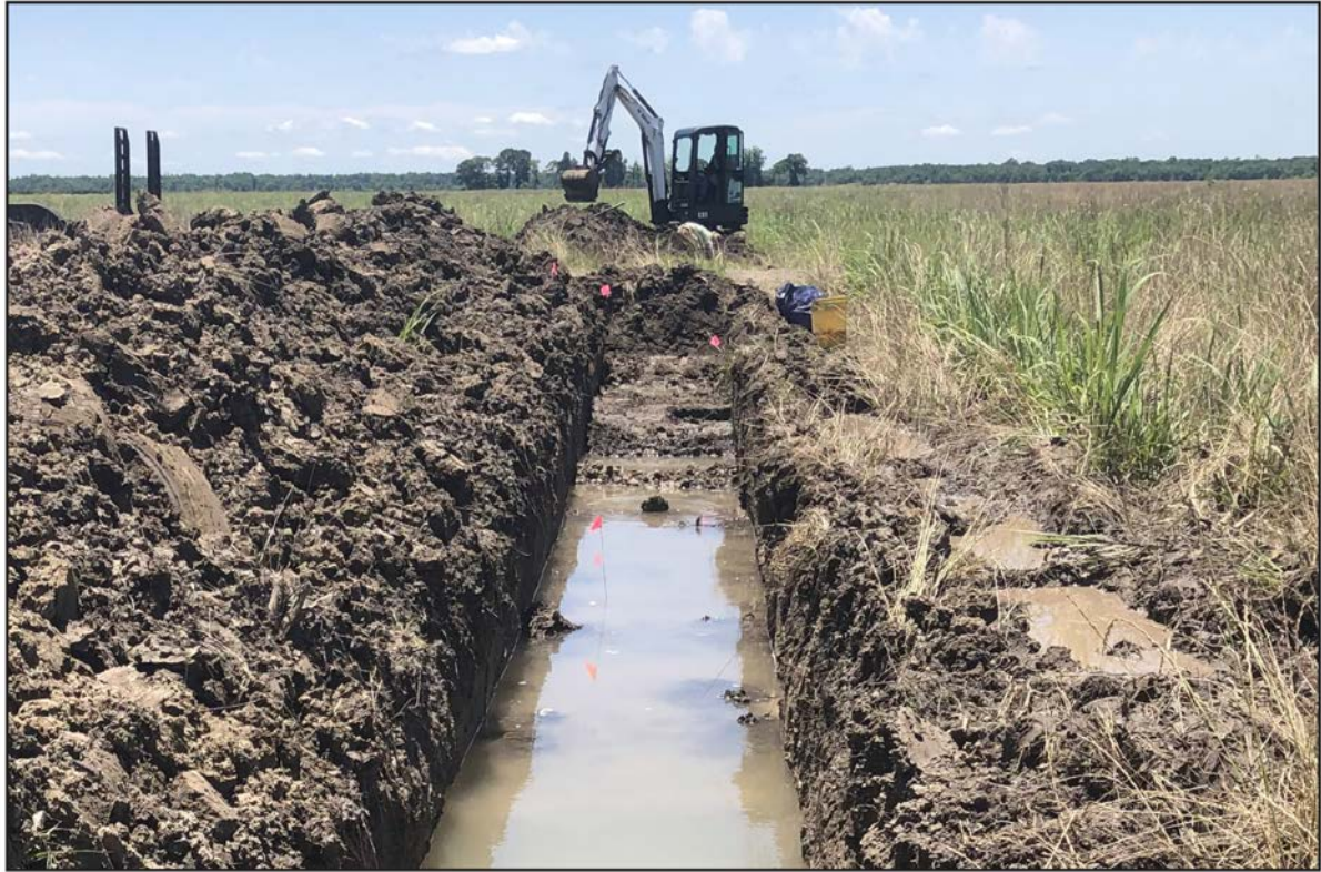
Figure 3-3. Photograph showing the flooded trenches being excavated by TerraXplorations, Inc., at the Buena Vista Plantation Cemetery in 2019 (after Jackson et al. 2019:Figure 6.1).
